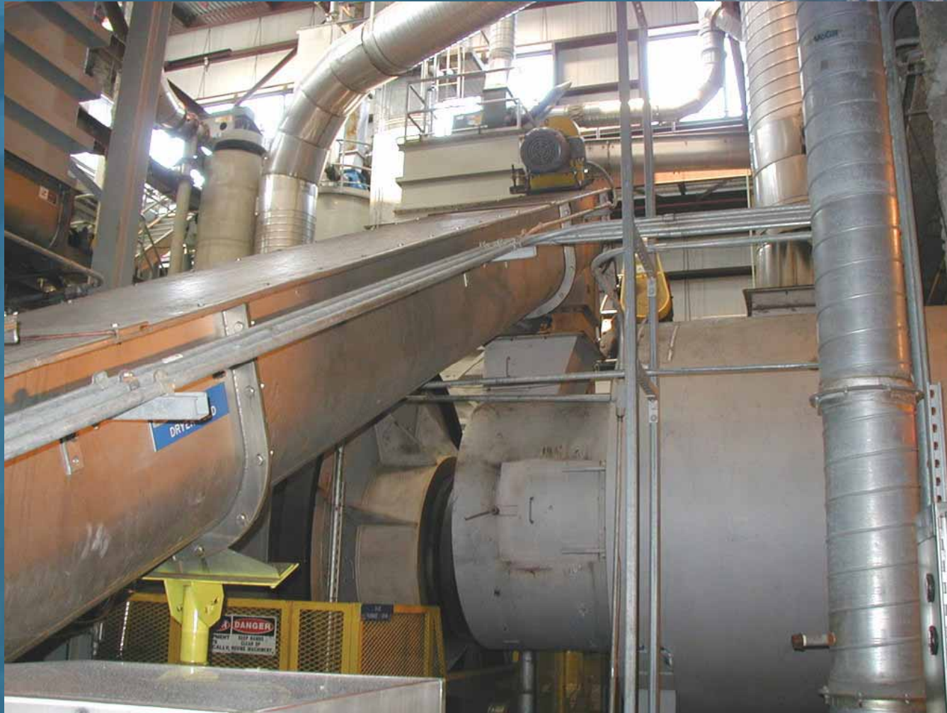
Biosolids feed line into an Andritz Direct Drum Dryer.
