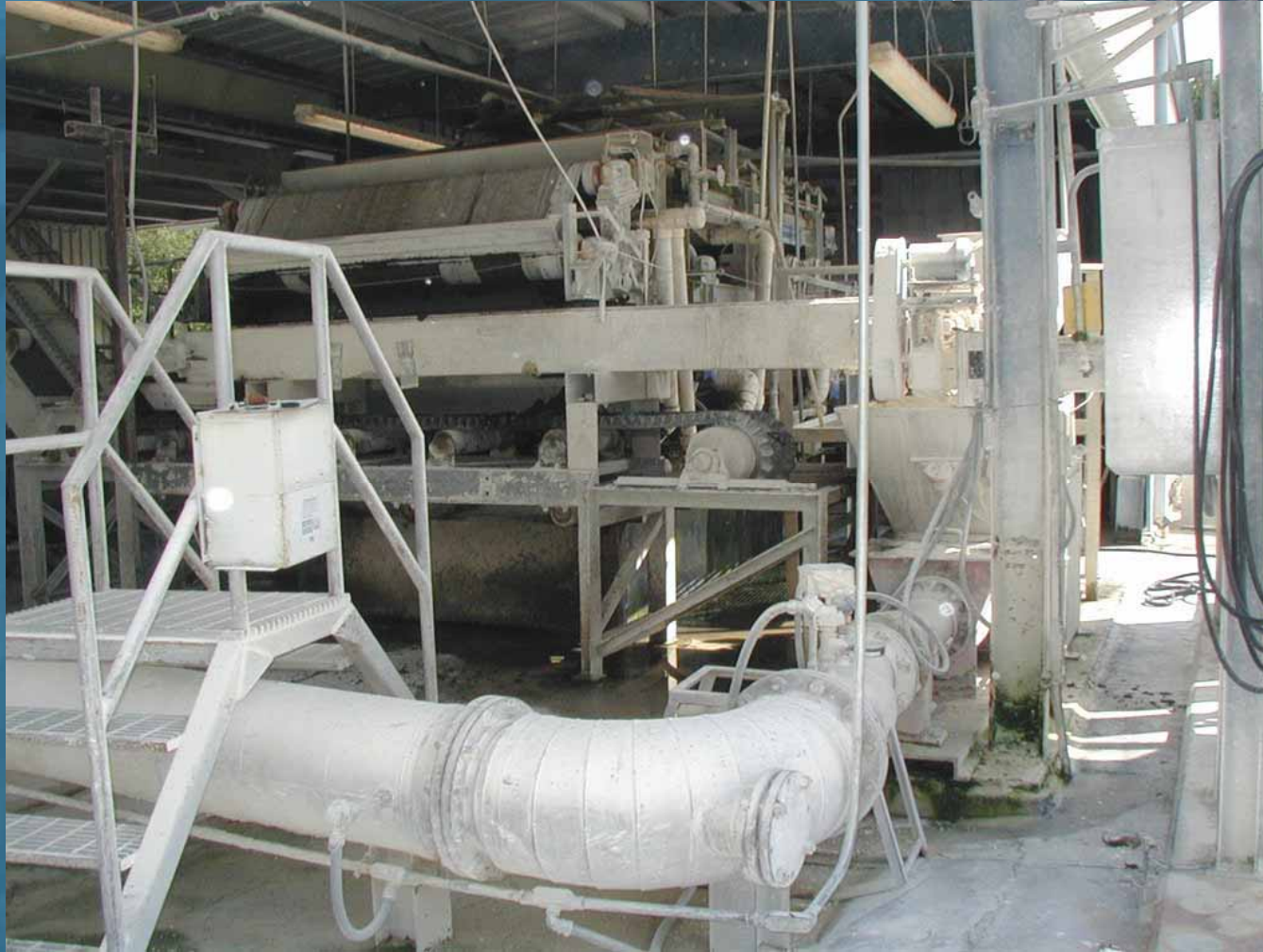
Bioset process (foreground) and belt press (background).
