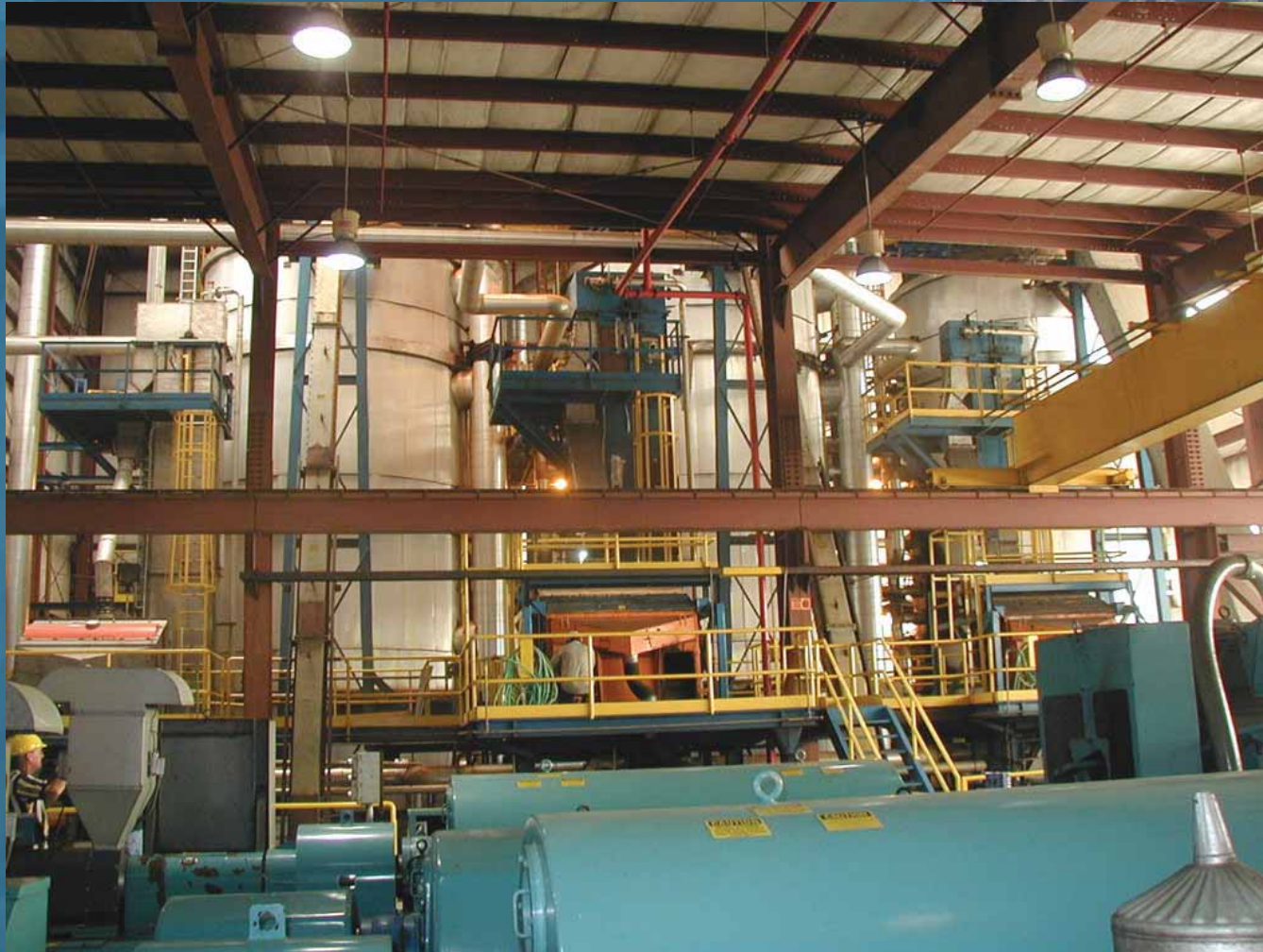
Centrifuges (foreground) and Seghers Pelletizers (background).
