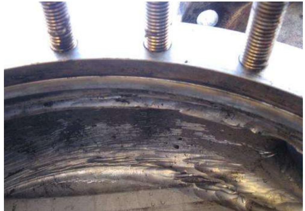
Discflo pump erosion
