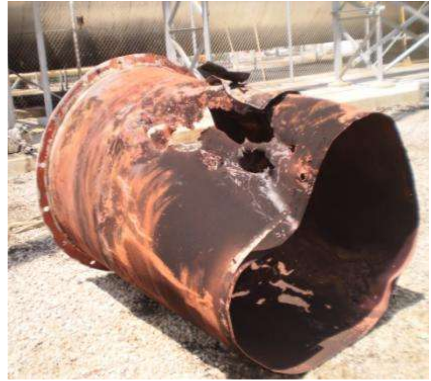
Cracked burner nozzle
